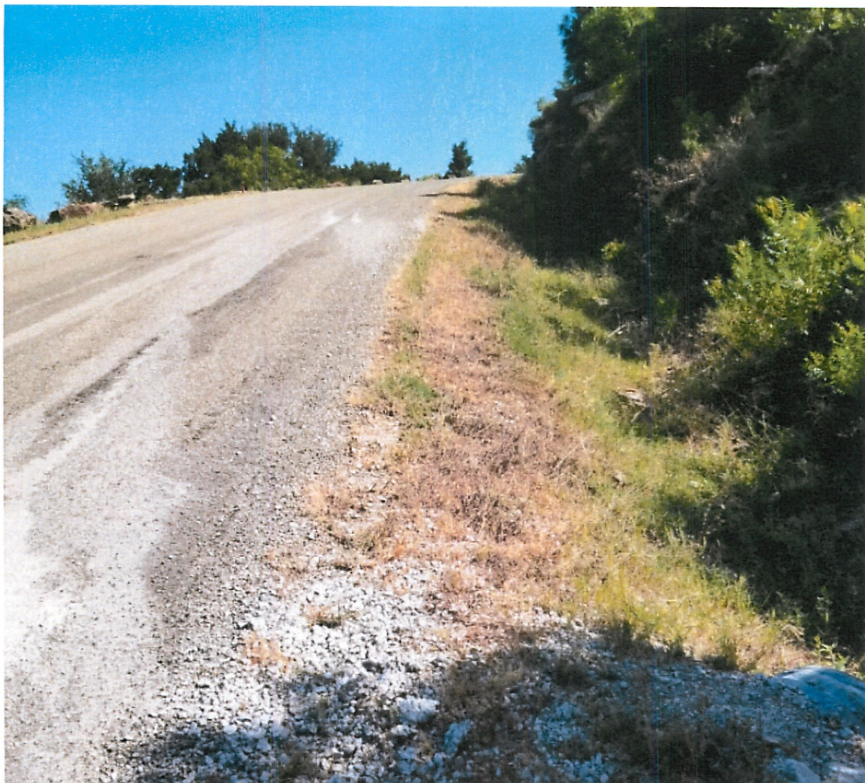
Unauthorized spraying on Wolf Creek Ranch Road (adj to MCW-1)
