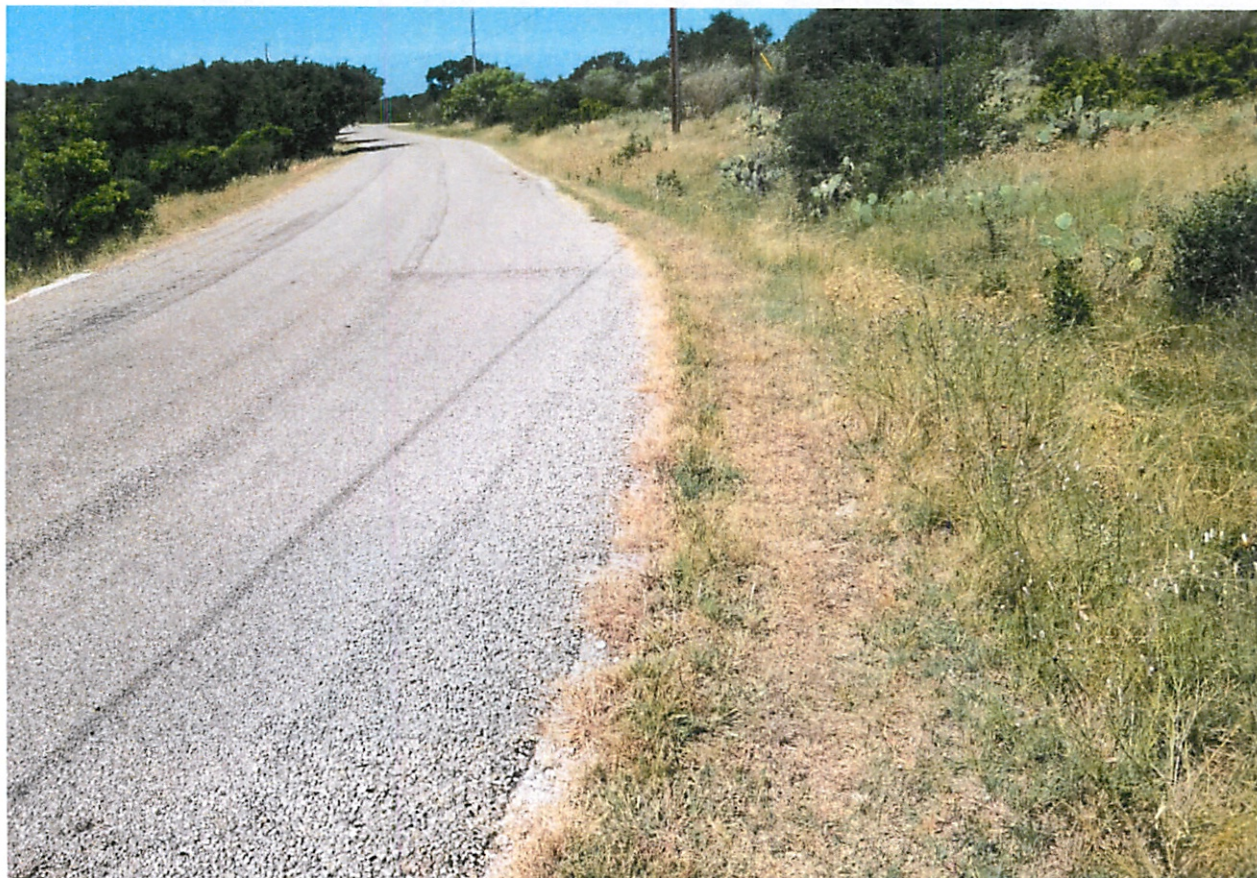
Unauthorized spraying on Wolf Creek Ranch Road (adj to MCW-5)
