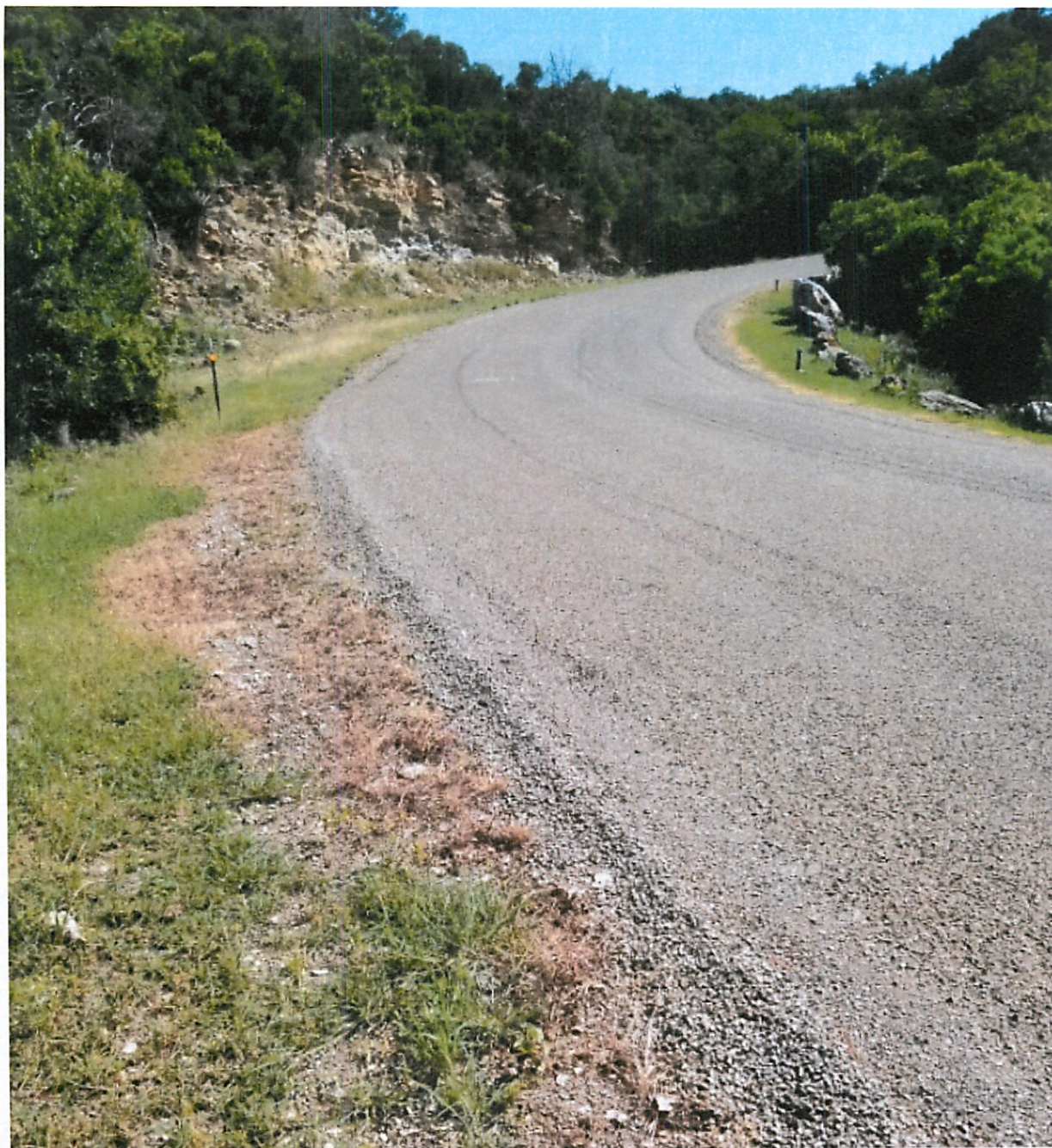
Unauthorized spraying on Wolf Creek Ranch Road (adj to MCW-4)
