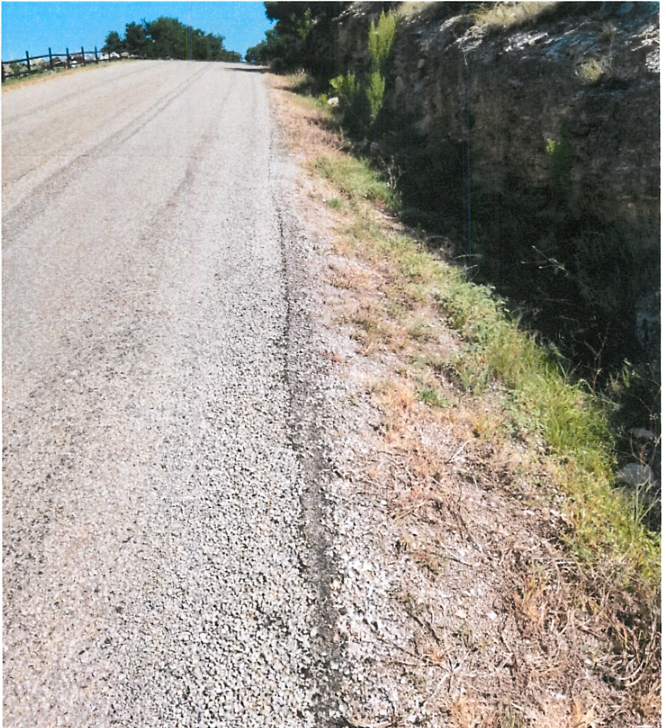
Unauthorized spraying on Wolf Creek Ranch Road (adj to MCW-2)
