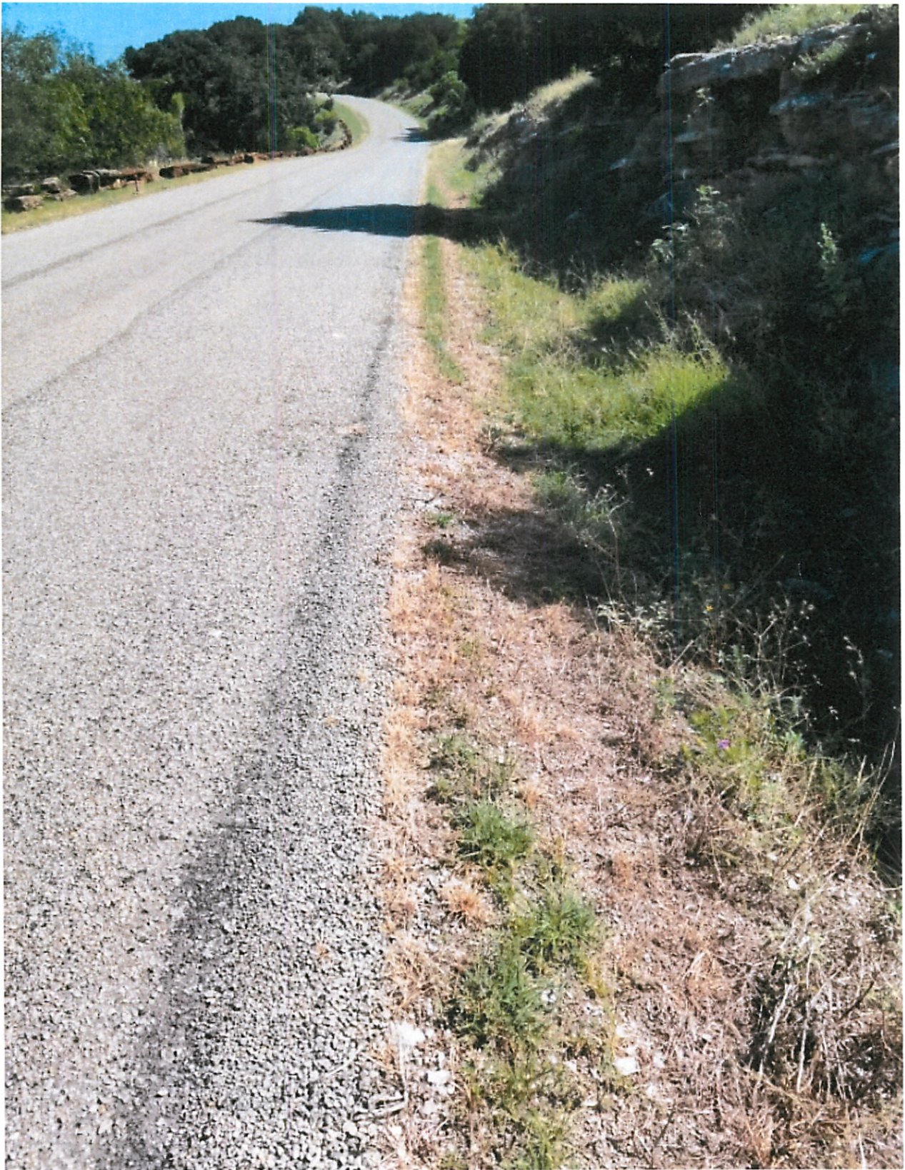
Unauthorized spraying on Wolf Creek Ranch Road (adj to MCW-2)
